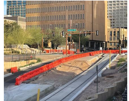
Valtir Rentals' 2001MB Barricades were used in the Phoenix Passenger Rail Project.
