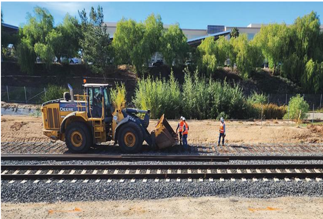
Hill International is overseeing construction on Metrolink’s Southern California Optimized Rail Expansion (SCORE), a $10-billion capital program benefitting regional passenger rail.
