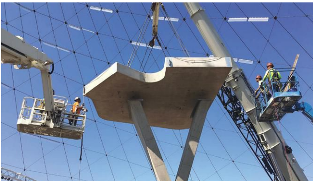
SENSORY EXPERIENCE Luminares light the structure (center); Garco Construction workers place a platform for the elevated walkway (bottom).
